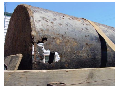
50 year old rusted heating oil tank
